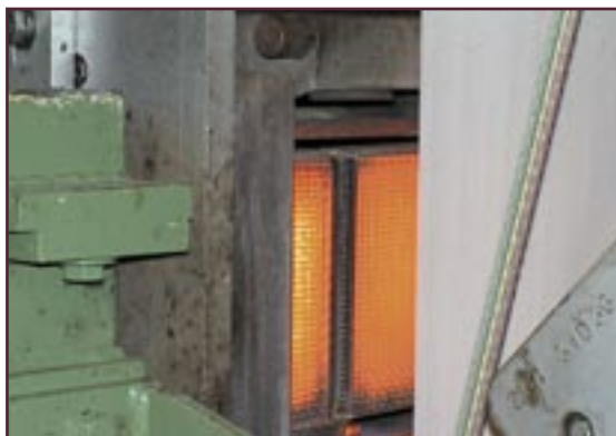
IR.D.S. emitters in operation on PM 3
